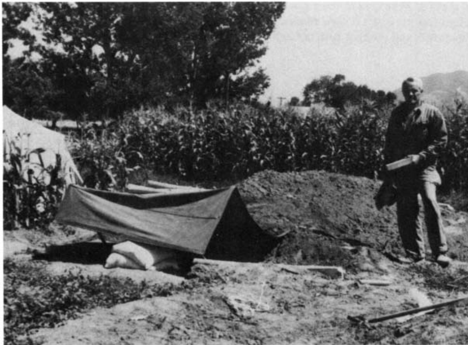
Fig. 5.6. Earth mounded over a 3½-foot-wide Pole-Covered Trench Shelter. The canvas canopy would protect the vertical entry against both fallout and rain. (A smaller canopy over the air duct-emergency exit at the other end is obscured by the mounded earth.)
